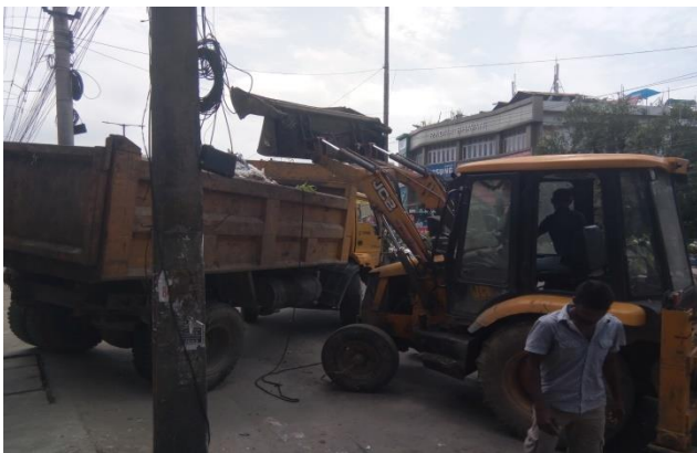
Fig.3.Loading of waste from the Primary Collection Point into the truck with the help of JCB
