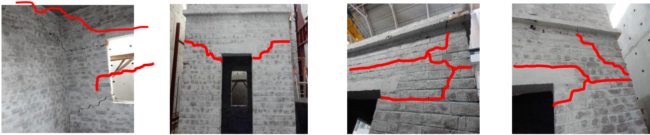
Fig. 3 Damage observed in the unstrengthened URM building in the form of cracks in different walls
