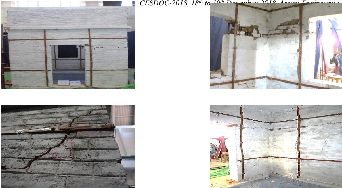
Fig. 6 Damage observed in the strengthened URM building in the form of cracks in different walls
