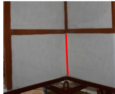
Fig. 8. An interface crack between the masonry wall and the main post after the entire testing events.
